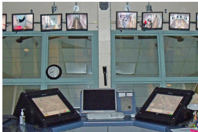
Multiple monitors are mounted in the Charlie housing unit at the Butte County Jail.
